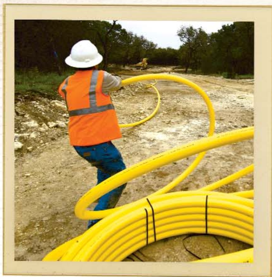
Reynaldo Carabajal, Construction and Maintenance Technician, uncoils piping at a construction site in New Braunfels, Texas.
