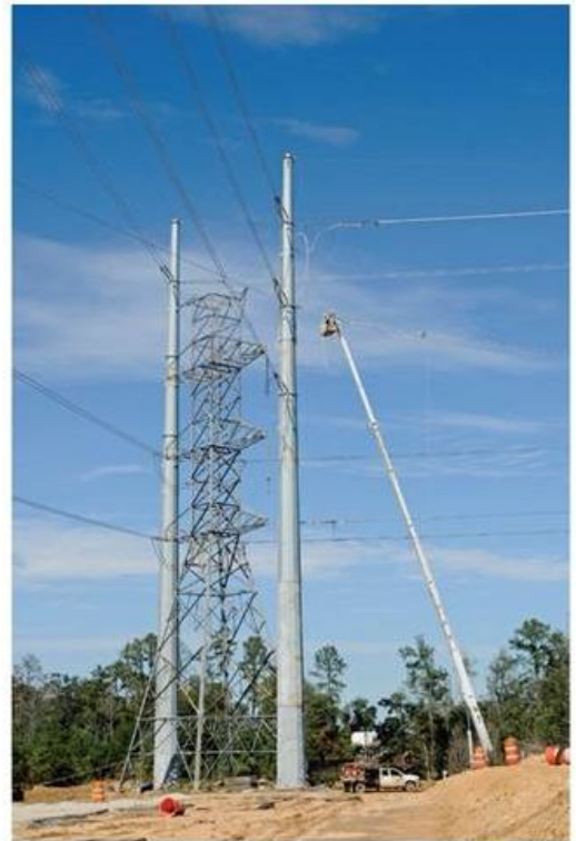
Raising high voltage transmission towers to accommodate new Highway US-99 corridor and serve load growth
