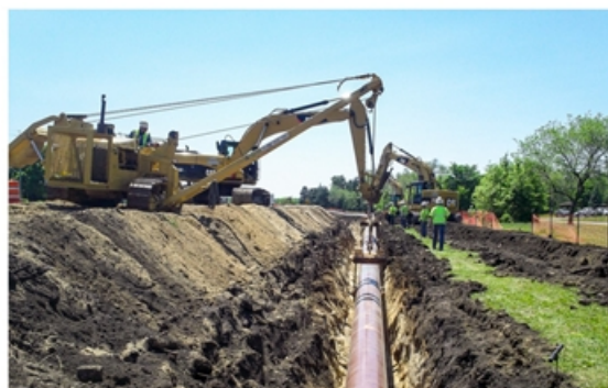
Work on the beltline project in MN – Infrastructure Services completing work for Natural Gas Distribution
