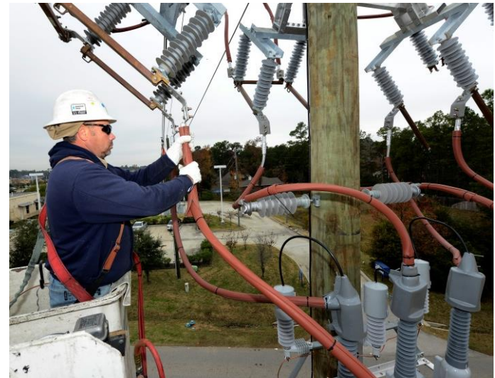
A Houston Electric lineman working on lines damaged by storms the week of April 17 th
