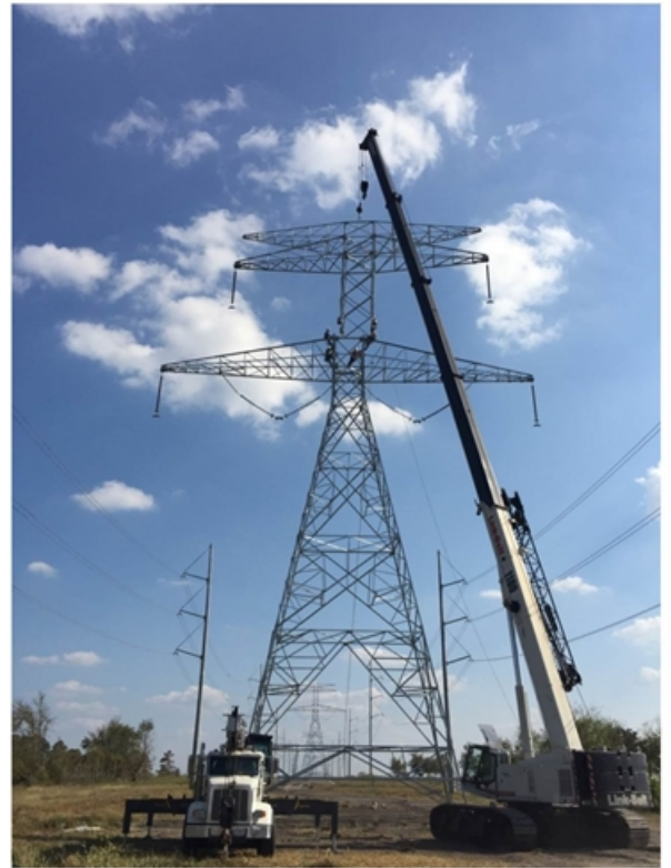
Construction of a new permanent 345kV double circuit tower in between temporary bypasses constructed to safely reenergize circuits damaged by tornadoes in April 2015.
