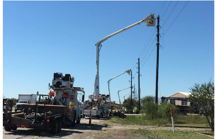
CenterPoint crews restoring power after a May 2017 “microburst” weather event in Sealy, TX
